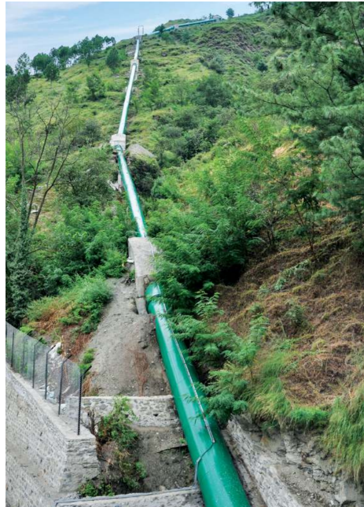
The discharge of Sarbari I is fed to Sarbari II through a pressurized tunnel and penstock of length approximating 3,851 meters.
