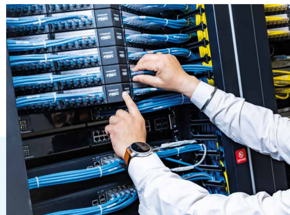
FLOVEL technicians often stay involved long after commissioning – with deep knowledge and dedication.
